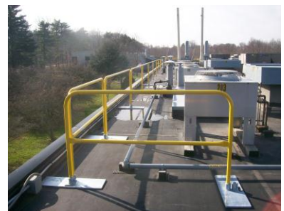
Guardrail systems, single point anchors and horizontal lifelines are examples of rooftop fall protection.
