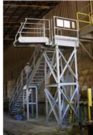
A stairway system with a gangway provides safe access to operations at height.
