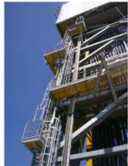
A series of ladder systems installed on an off-shore oil rig
