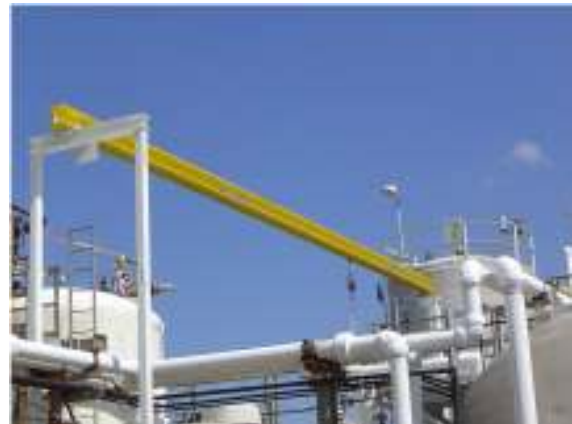
A rigid trolley beam system used while performing instrumentation on a tank at a refinery facility.
